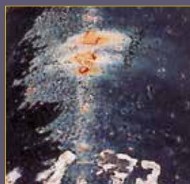
Non-zinc coated: the damage is worsened and the corrosion (red marks) extends beyond the notch
